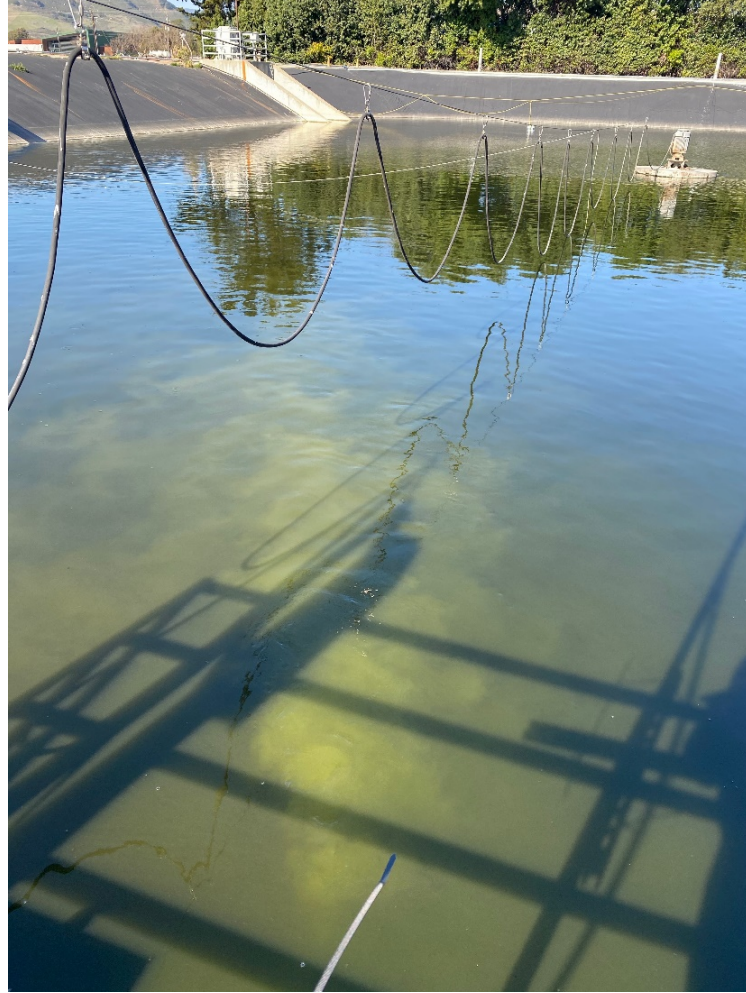
FIGURE 24 EMULSIFICATION OXYGEN FLOW IN TO SUPERNATANT LAGOON AT SLO WRRF
