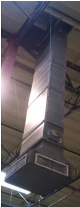
Ductwork before the retrofit
