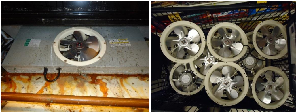
FIGURE 3 - RETROFIT PMSM FANS AT THE HOST SITE
