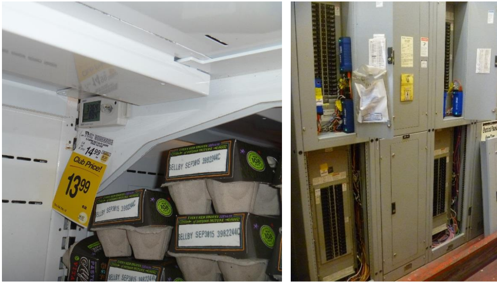
FIGURE 7 - CASE AIR T/RH AND ENERGY LOGGERS AT FAN CIRCUIT PANELS
