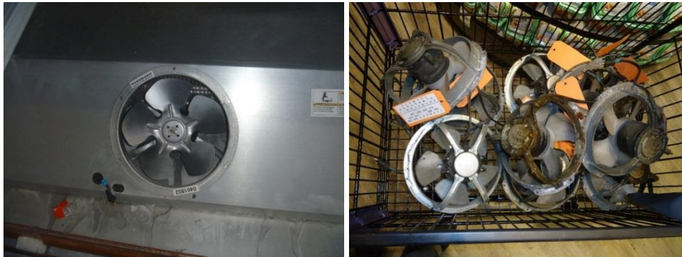
FIGURE 2 – INCUMBENT BASELINE FANS AT THE HOST SITE
