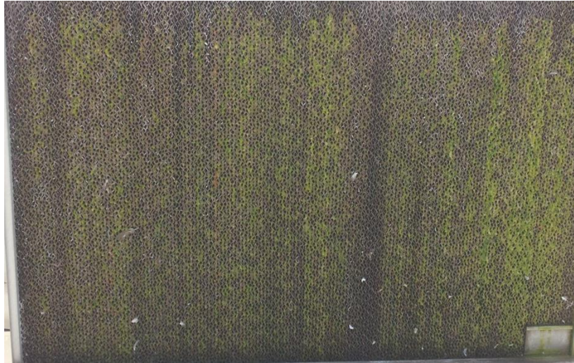
FIGURE 34 – ALGAE GROWTH AND CALCIUM BUILD-UP WAS OBSERVED ON THE DIRECT EVAPORATIVE COOLING MEDIA
